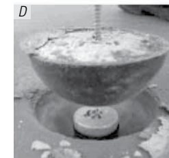
D – The recess former is removed leaving a clean void and the collet, which is easily pulled off to allow the clutch to engage on the anchor.
