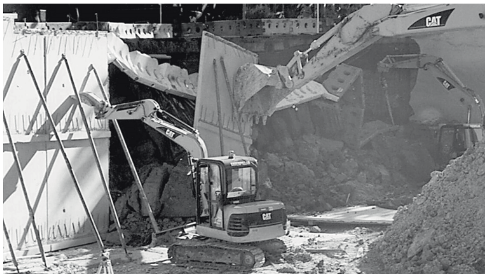
A complex series of errors – site preparation, incorrect bracing
