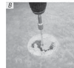
B – Using a self-drilling hex head wood screw and electric drill, drill into the centre of the recess former.
